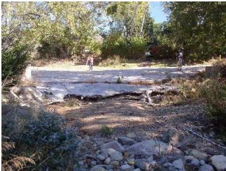
Bonsall Drive Arizona Crossing. Example of one barrier in study area. Photo from CalTrout 2006 report.
